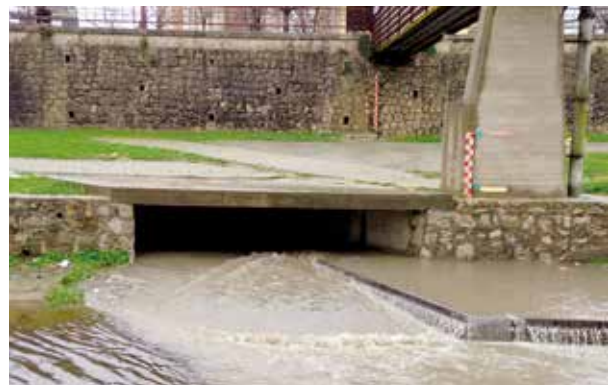
CSO overflowing rain and WW
